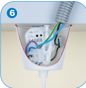
Installation of the actuator in the light fixture
