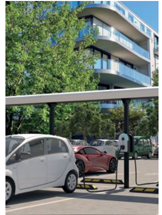
Outdoor Charging Infrastructure
