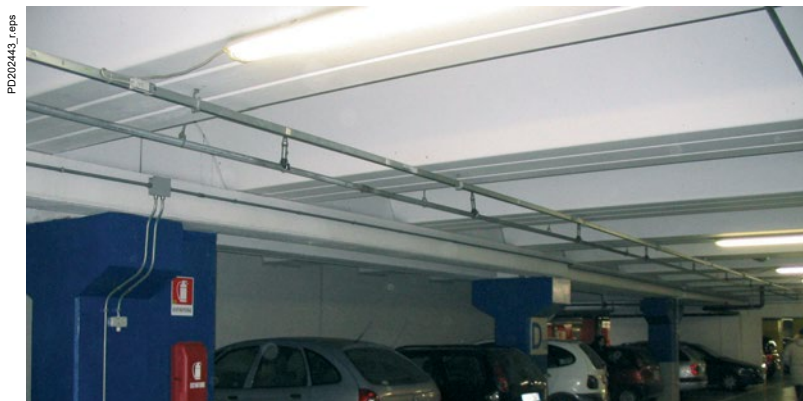
Canalis KBA supplying luminaires nearby sprinklers.
