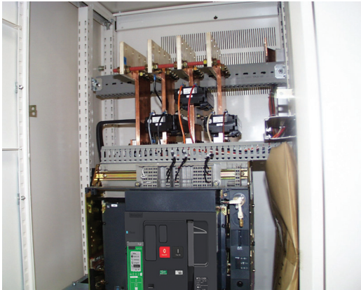
CT on vertical busbars.
