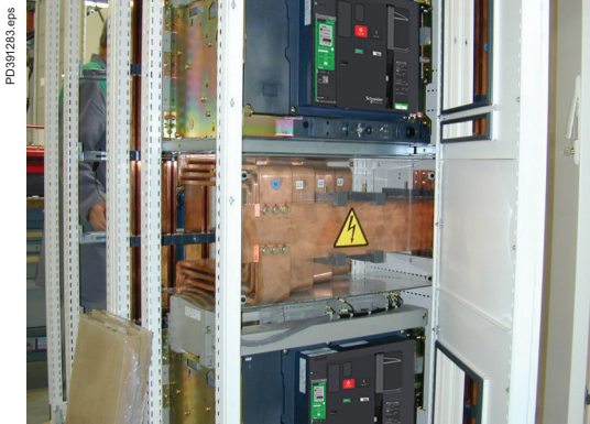
Source changeover system in the same cubicle.
