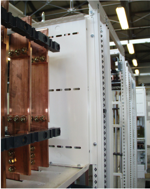
Dismountable vertical busbars.
