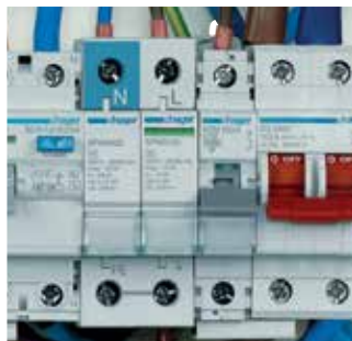
VA02SPD installed inside a consumer unit
