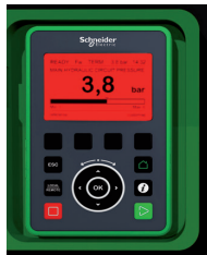
Detected fault: Red screen when there is a detected error
