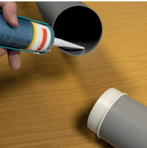
Apply a smooth layer of non hardening sealant/acrylic around the inside edge of the second piece of ducting
